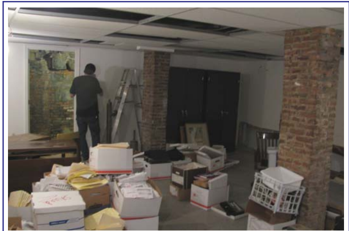
The summer renovation of the MACo offices is nearly complete after extensive renovations to the HVAC system, the installation of a sprinkler system, and remodeling the basement of the building to add office space. Meetings in the library on the second floor are expected to resume later this month.
